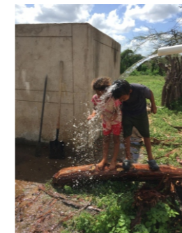
Kenya 7.5kw Pumping system
