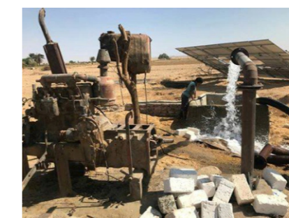
Yemen 55kw Pumping system
