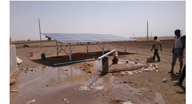
Ethiopia 9.2kw Pumping system
