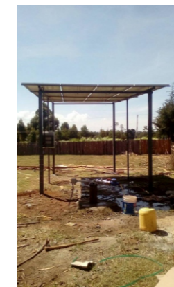
Kenya 2.2kw Pumping system
