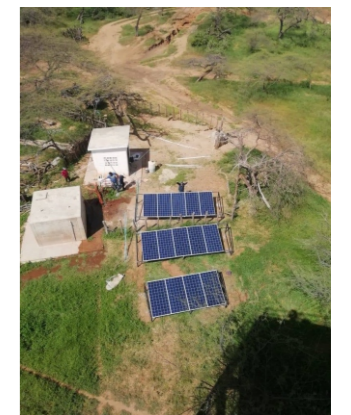
Cambodia 5.5kw Pumping system
