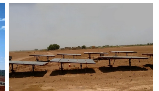
Pakistan 30kw Pumping system
