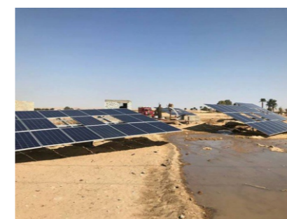
Egypt 45kw Pumping system
