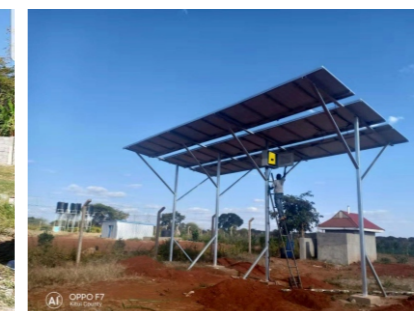
Kenya 13kw Pumping system
