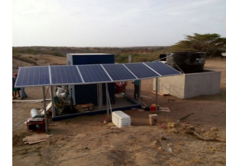
Colombia 2.2kw Pumping system
